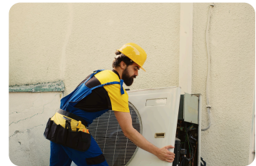
AC, HVAC & CCTV Maintenance
